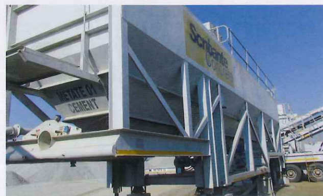
Batching is automated via the control room, through a series of augers and pumps which feed pre-determined amounts cement, fly-ash and water to the batch mixer
